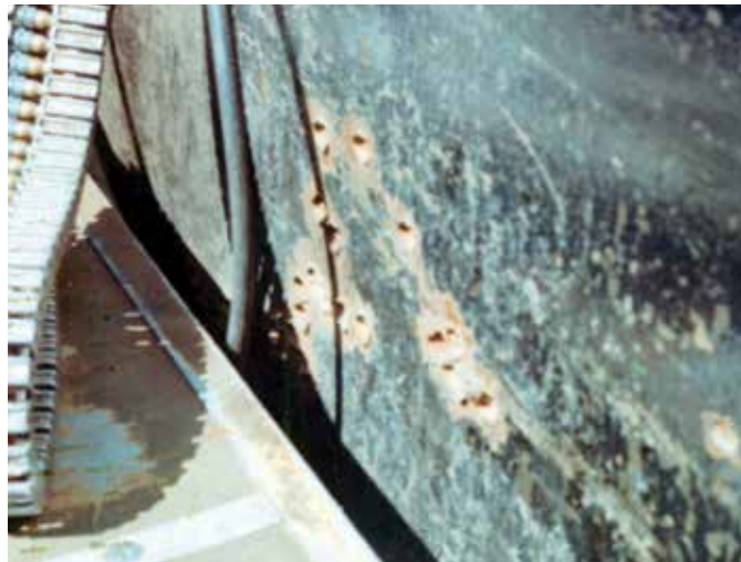
Damage caused by shrapnel bounding off the wall.
